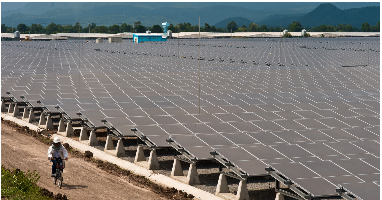
Thailand's 73-megawatt Lopburi solar power plant is the largest solar photovoltaic project in the world, and central to the country's efforts to generate energy from renewable sources. Photo by Gerhard Joren. ADB Photo Library.
